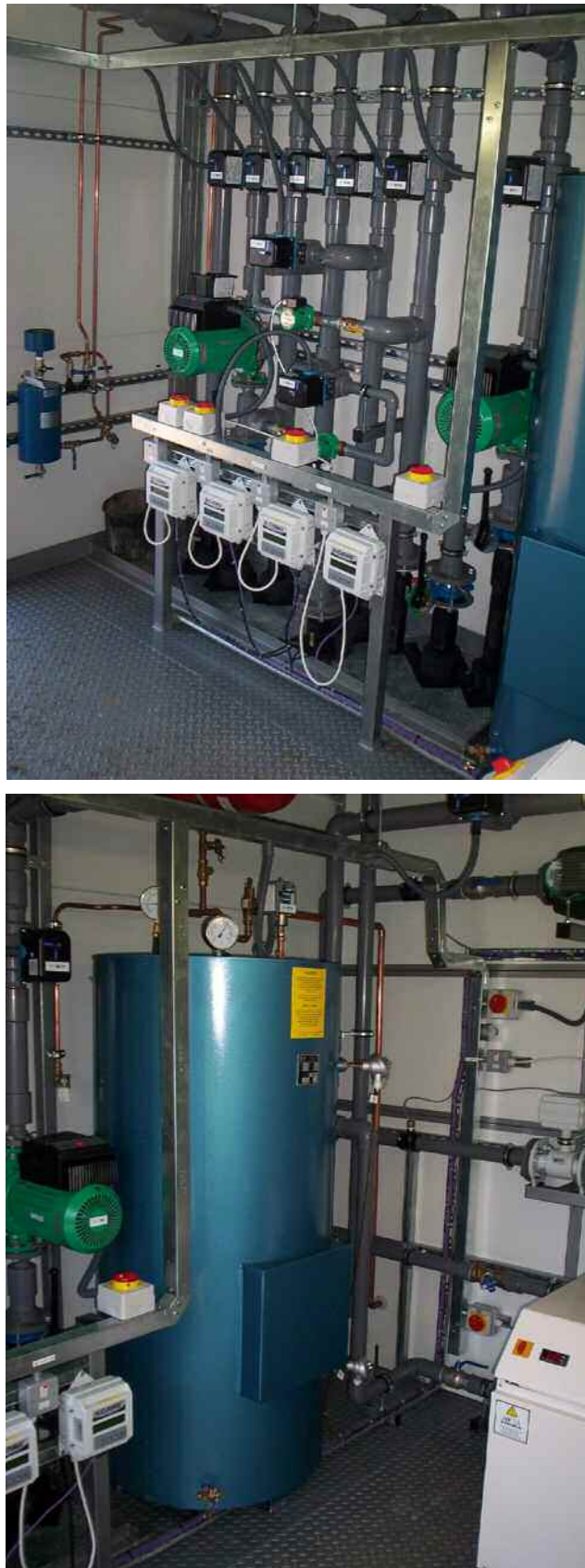
Figure 6.1. Photographs of the inside of the pump house
